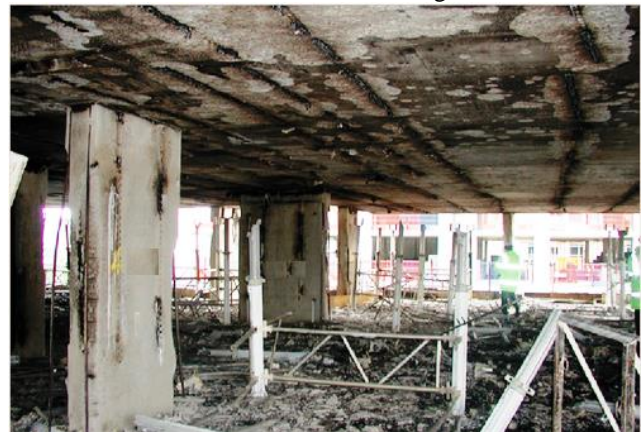
Figure-1. Concrete failure with time
